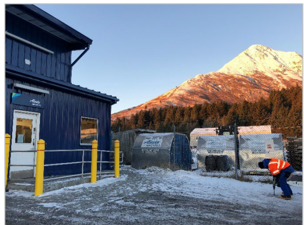
Exhibit 2-1: Field staff use a rotary drill to sample the asphalt profile outside the Alaska Air Cargo building at the ADQ.
